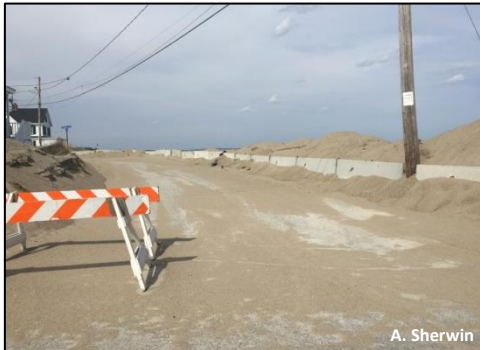
Coastal road in the Camp Ellis neighborhood of Saco covered with sand from adjacent beach due to wind and storm overwash.
