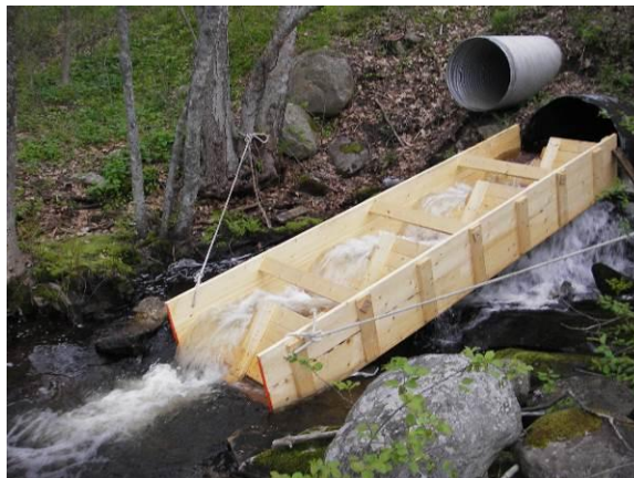
Improperly installed culverts can impede movement and restrict habitat connectivity for many aquatic ecosystems. In this case, a fish ladder may allow some species to traverse the barrier. © Department of Marine Resources
