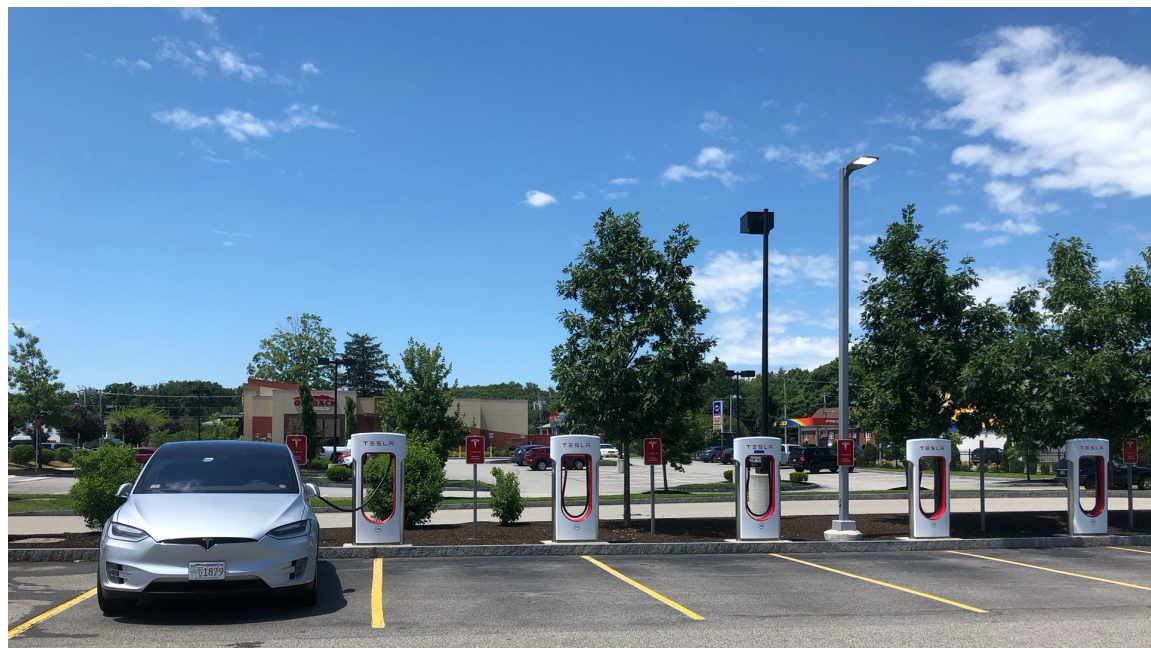
A bank of EV Superchargers in Seabrook, NH. Photo: Tom Morgan
