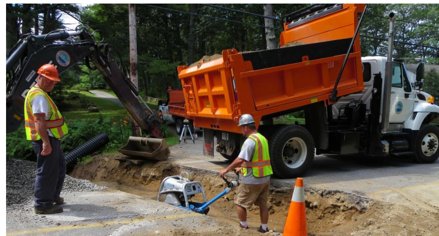
Culvert replacement on Turbats Creek Road. Photo courtesy of the Public Works Department
