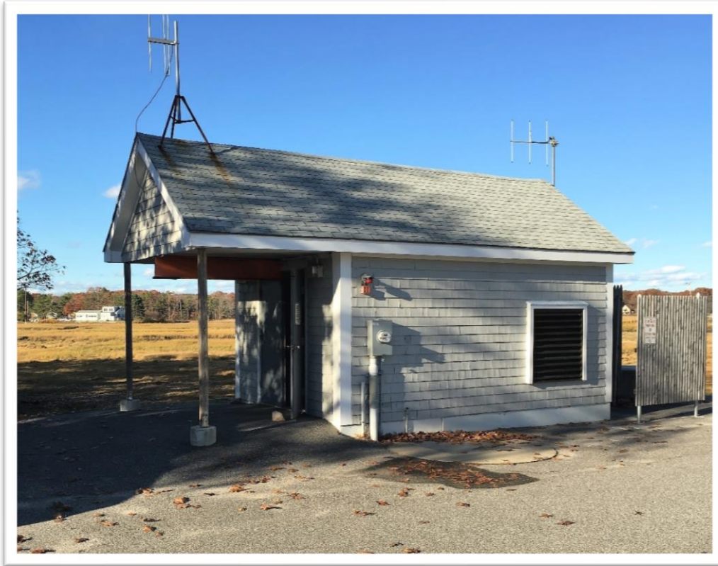
FIGURE 12 –KING’S HIGHWAY-MAIN PUMP STATION
