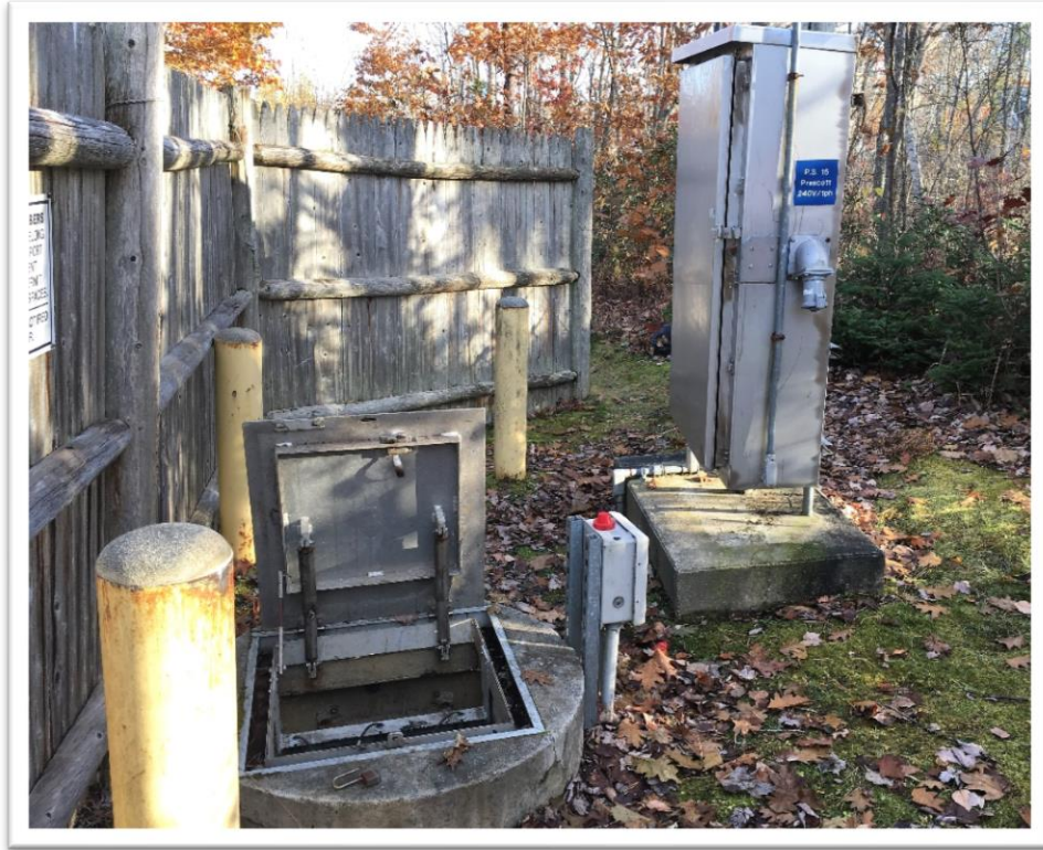
FIGURE 15 – PRESCOTT DRIVE PUMP STATION
