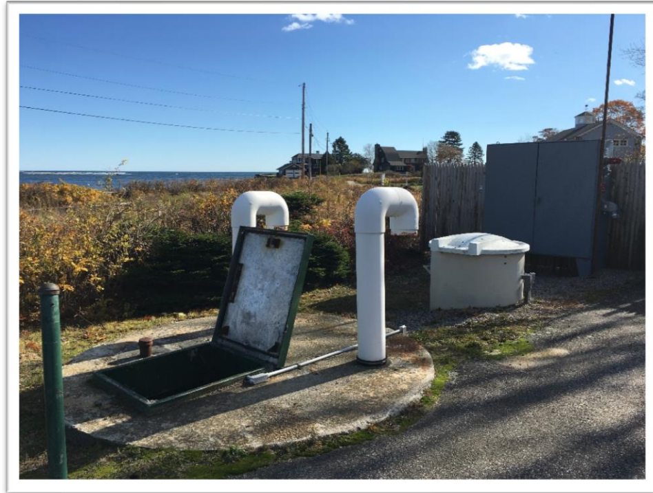
FIGURE 7 – TURBATS CREEK PUMP STATION
