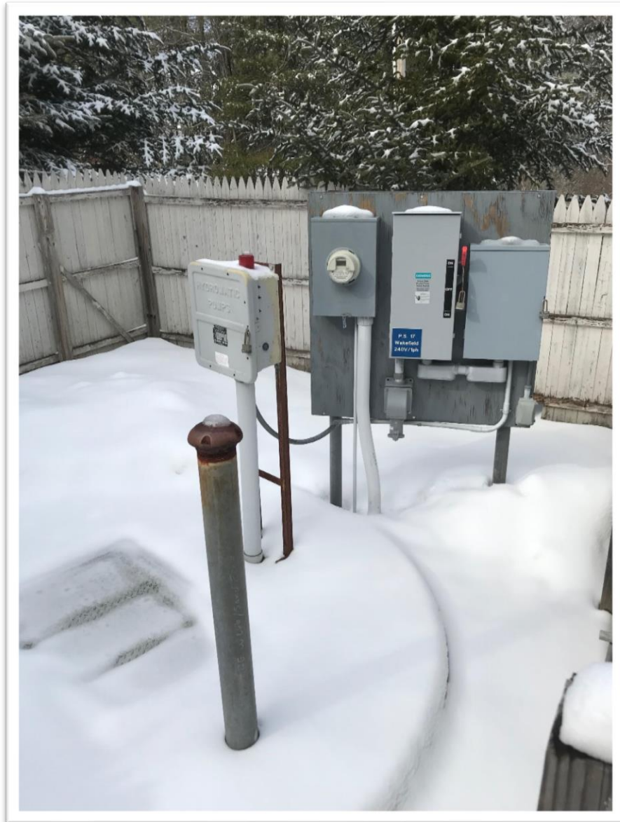
FIGURE 17 – WAKEFIELD PASTURE ROAD PUMP STATION
