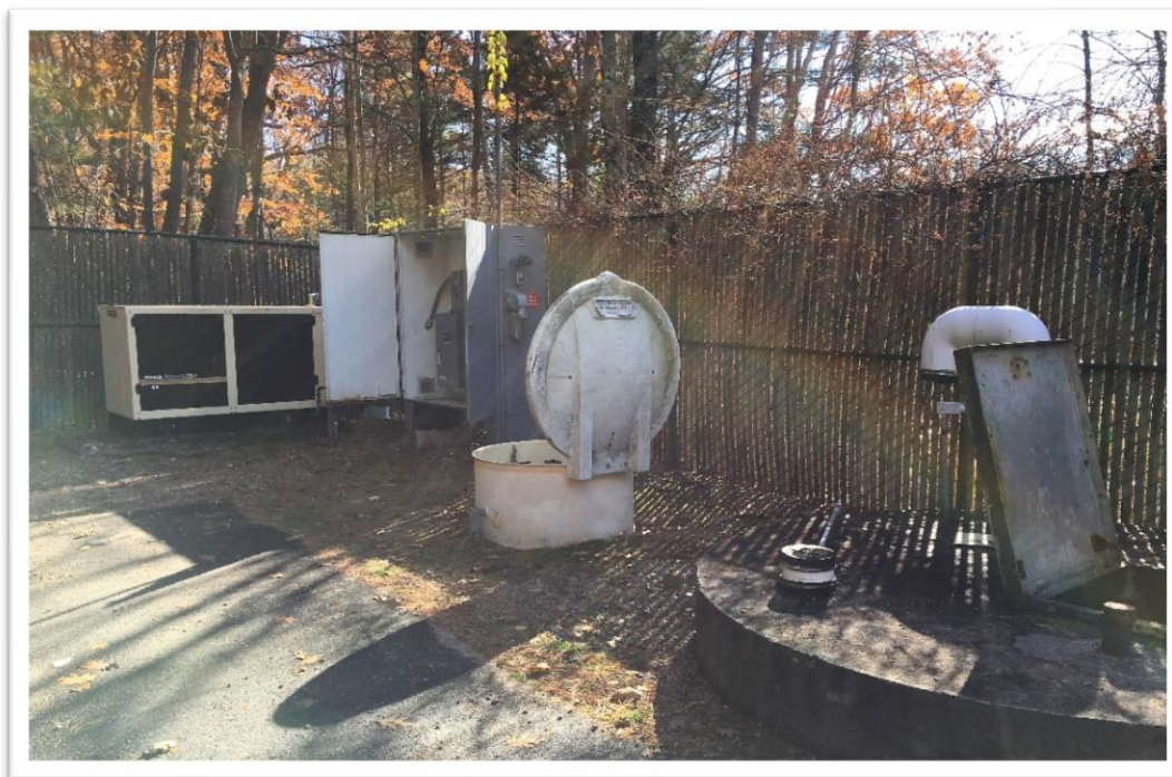
FIGURE 8 – WILDES DISTRICT ROAD PUMP STATION
