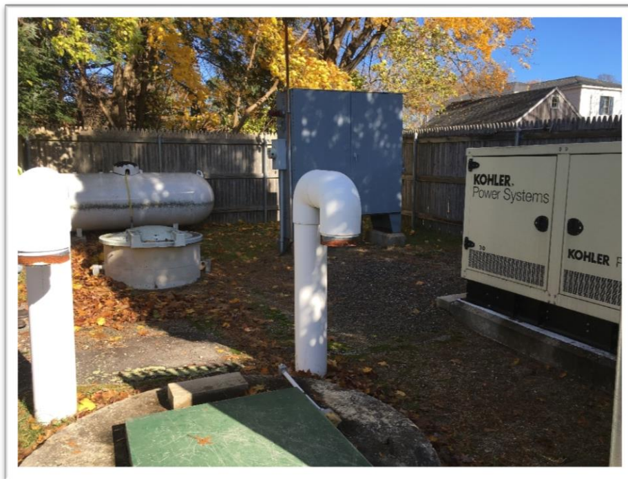
FIGURE 2 – MILL LANE PUMP STATION
