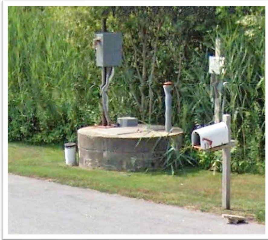
FIGURE 16 – WASHINGTON COURT PUMP STATION
