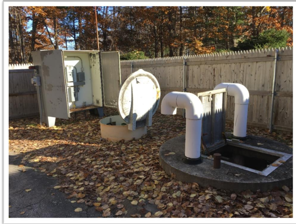
FIGURE 11 – MILLS ROAD PUMP STATION
