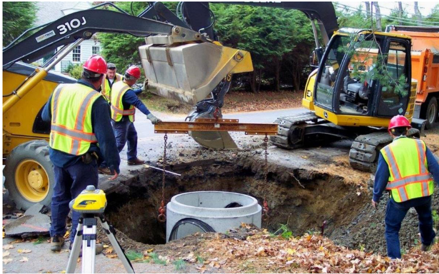
Stormwater drainage and sidewalk construction on North Street. Photo courtesy of the Public Works Department.
