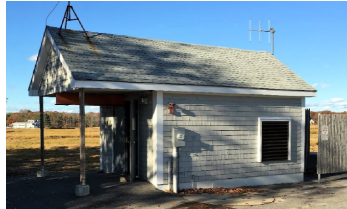
Pump Station #12, King's Highway. Photo: Wright-Pierce.
