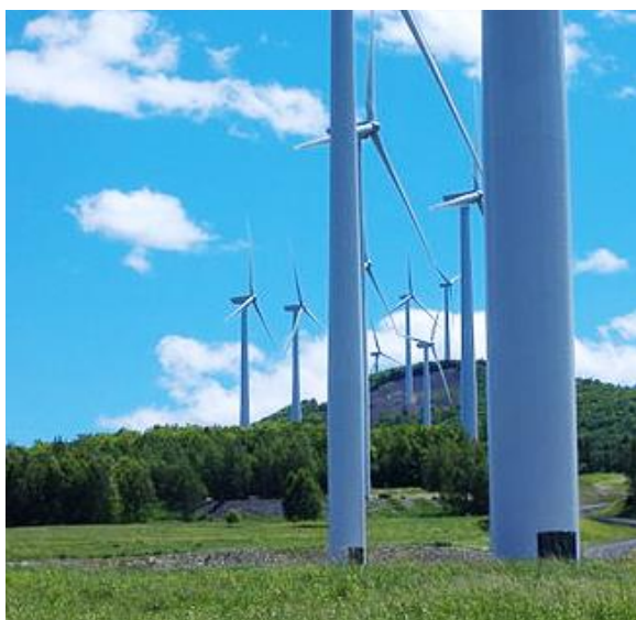
Several of the twenty-eight 1.5 MW wind turbines at the Mars Hill Wind Farm in the Saint John valley. Photo: Michael Surran.
