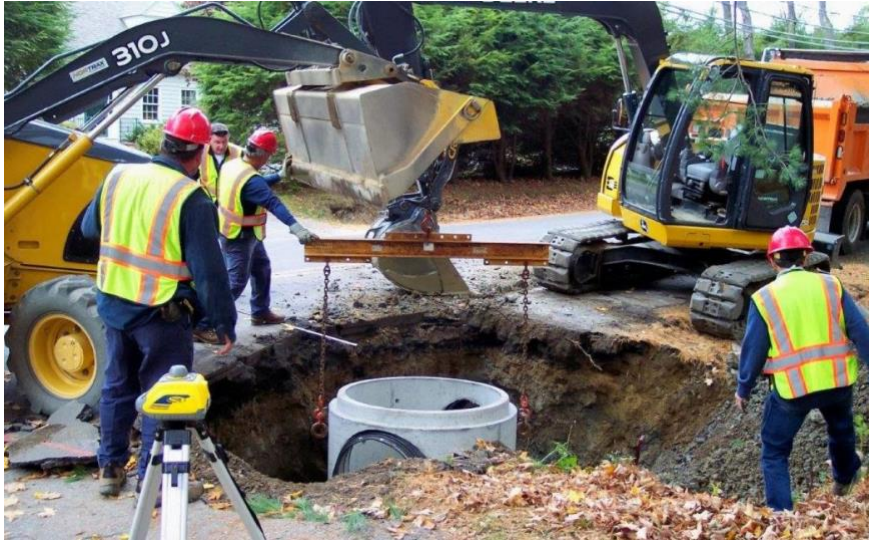
Stormwater drainage and sidewalk construction on North Street. Photo courtesy of the Public Works Department.
