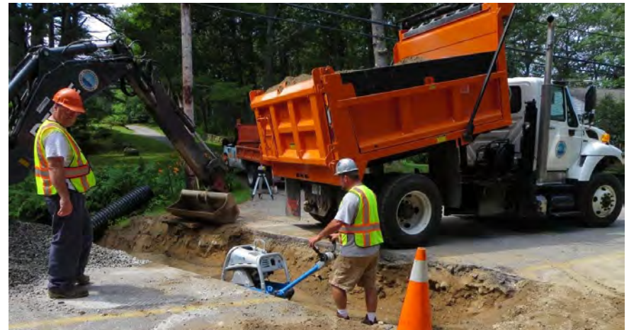
Culvert replacement on Turbats Creek Road. Photo courtesy of the Public Works Department.
